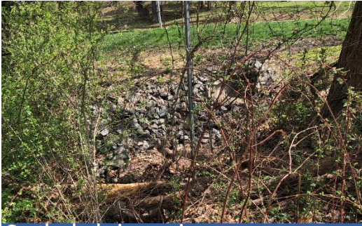
Southerly drainage pipe
