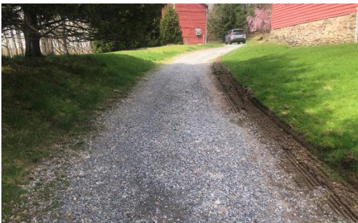
Evidence of obsolete driveway width
