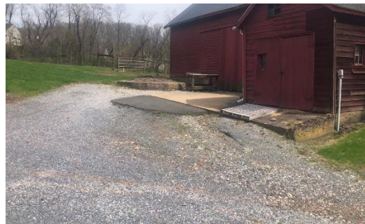
Evidence of erosion
